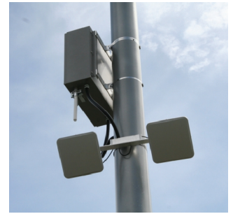
Outside the terminal, Motorola’s XR Series RFID readers are installed outside the terminal in NEMA enclosures to ensure reliable operation in sub-zero temperatures — a critical requirement for the Quebec-based transit system.
